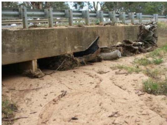
Figure 4. Sediment impact on bridge and road infrastructure
